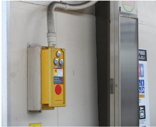
Fig 5.10 Emergency stop button in station
