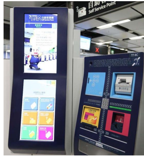
Fig 5.7 Staff machine in MTR Whampoa Station
