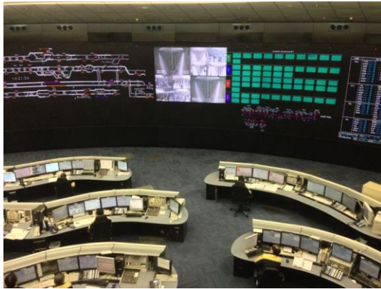
Fig 5.25 Central monitoring center
